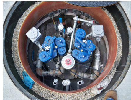
Twin Variable Speed STP Pumps Ratio the Blended Product Into the Diesel
